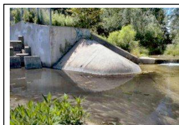
Polluted (black) sediment deposit at a stormwater outfall
